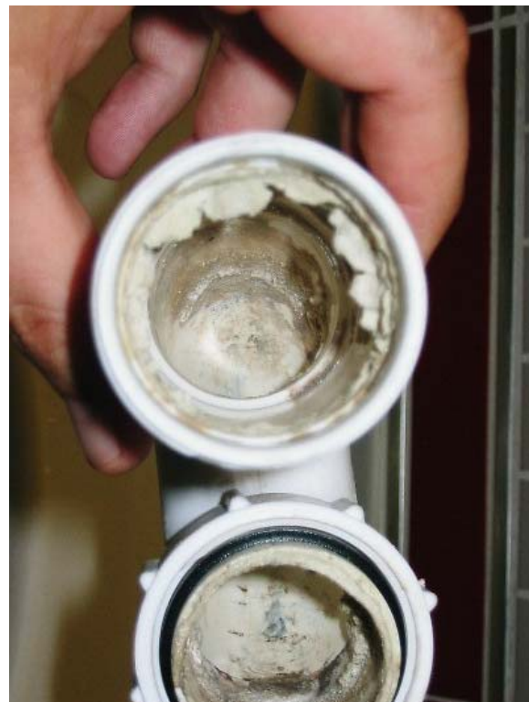
The same pipe-work after 6 months using Biological Toilet Blocks TOSS BLOCKS®
